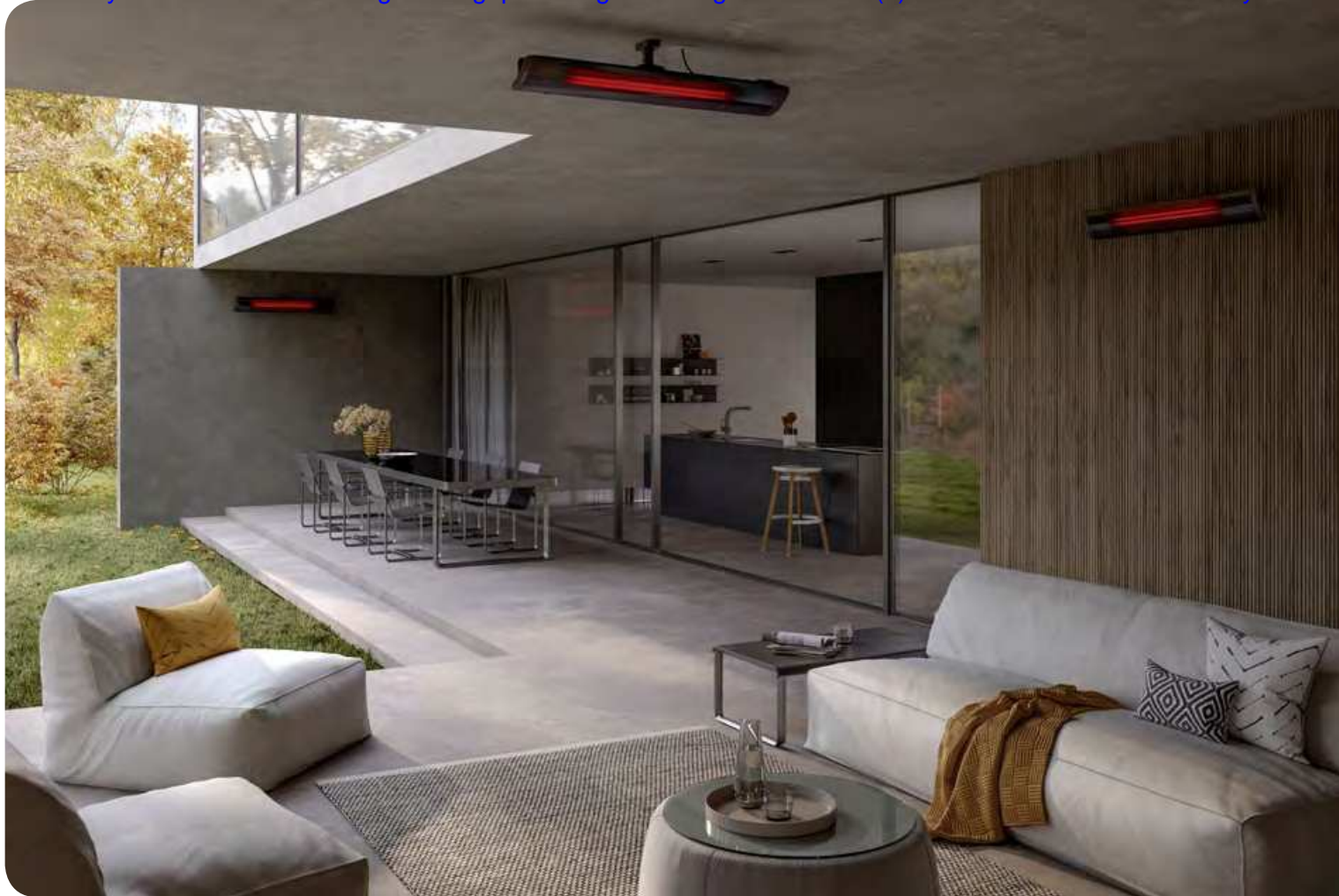
HEATSCOPE® PURE design heater · Terrace installation, Münster · Germany
